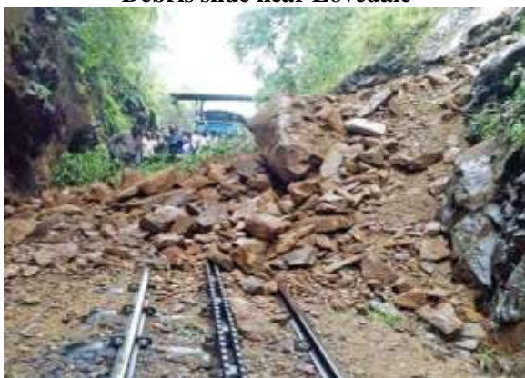
Rock fall along railway line of Coonoor – Mettupalayam road
